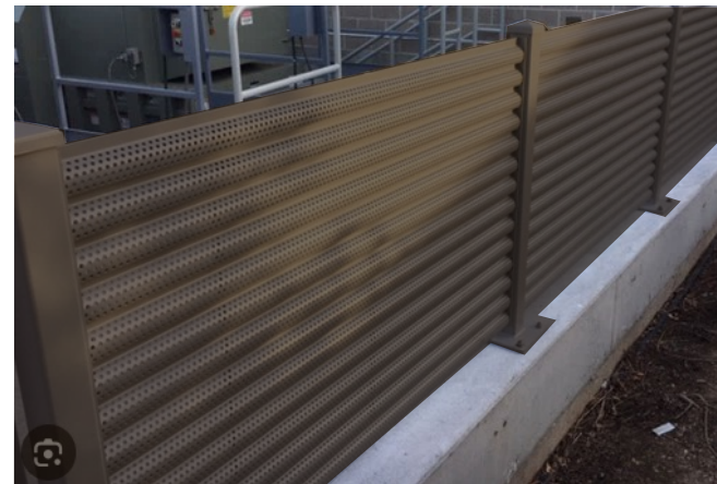
Screening of Pump Station Equipment
